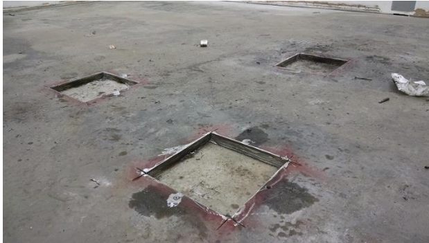
Example of shielding application that amplified vibrations. The shielding was comprised of aluminum, silicon steel, and low carbon steel. The shielding had to be cut to create pads for the equipment allowing the equipment to sit directly on the concrete slab. This resolved the vibration issue, but reduced the effectiveness of the shielding.
