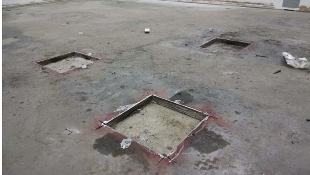
Example of shielding application that amplified vibrations. The shielding was comprised of aluminum, silicon steel, and low carbon steel. The shielding had to be cut to create pads for the equipment allowing the equipment to sit directly on the concrete slab. This resolved the vibration issue, but reduced the effectiveness of the shielding.
